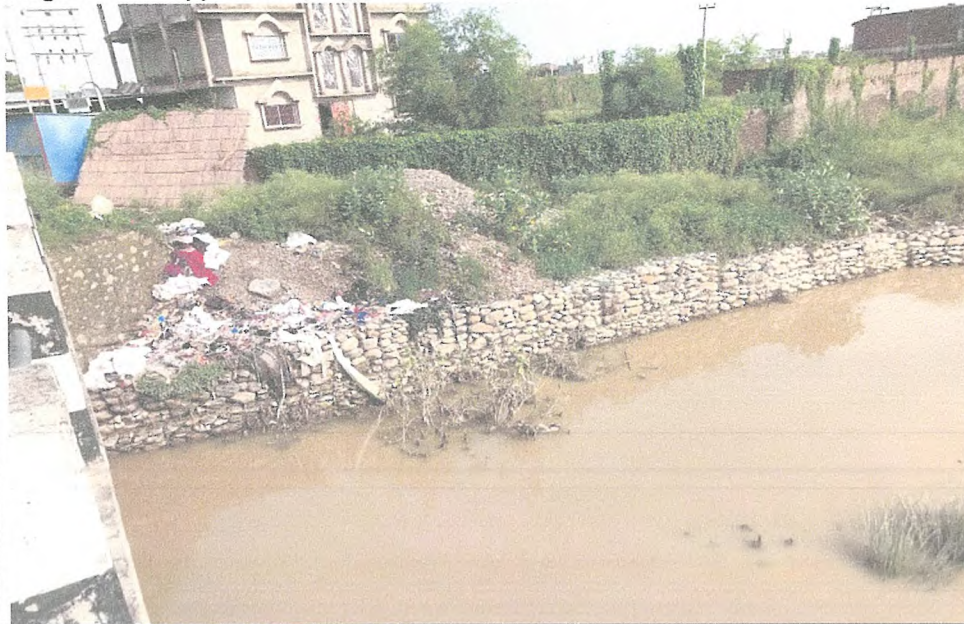
Stage-4 Overtopped and plugged Outfall no.-9
