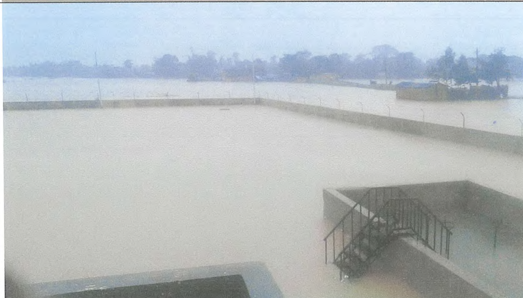
Water level raised more than half of 1.2 m high boundary wall inside STP
